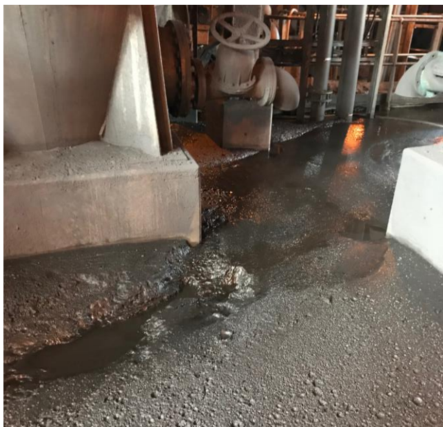
Figure 1: Sumps filled with spilt magnetite
